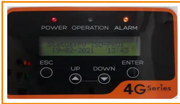
Figure 5: The PV system has a low impedance problem
