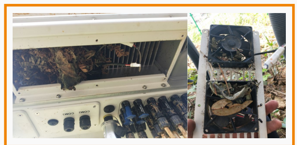
Figure 1: The accumulation of fallen leaves blocks the cooling air ducts and fans
