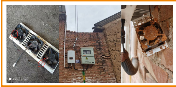
Figure 2: Rodent bites the fan cable, and the sand gets stuck on the fan
