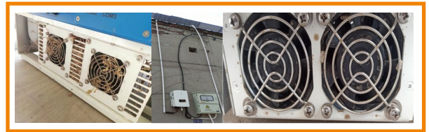
Figure 3: Debris blocks the inverter air ducts and fans, causing inverter failure
